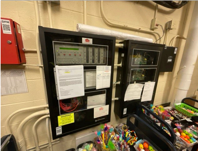
19 - FIRE ALARM SYSTEM
